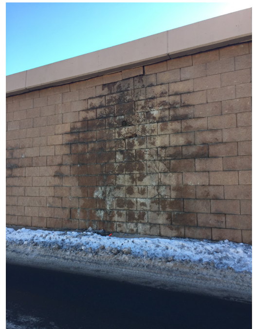
I-70/ Carr Street MSE wall damage
